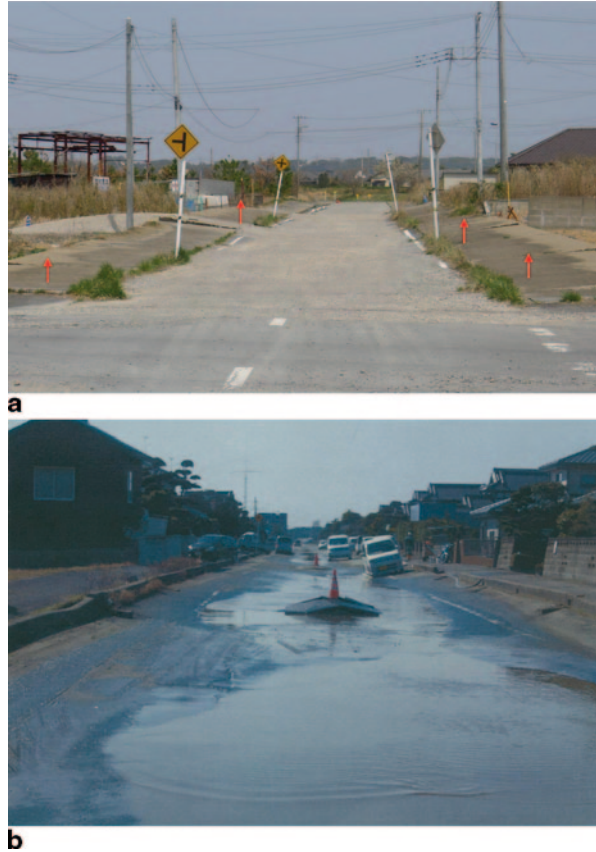
Fig. 36 Damage to the road in Horiwari, Kamisu. a Settlement of the road with the walkway that had moved toward the center. b Floating up of the buried water-drainage channel on both sides of the road
