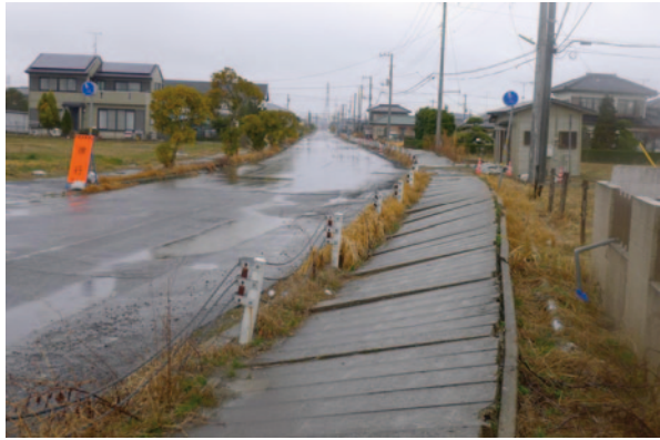
Fig. 16 Outward distortion of the box-type buried drainage channel installed along the roadside at the site A in Fig. 13—A view to the northeast
