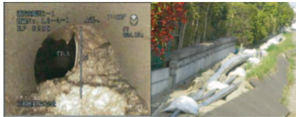
Fig. 1 Clogging and floating of sewage pipes. (From website of Urayasu City)
