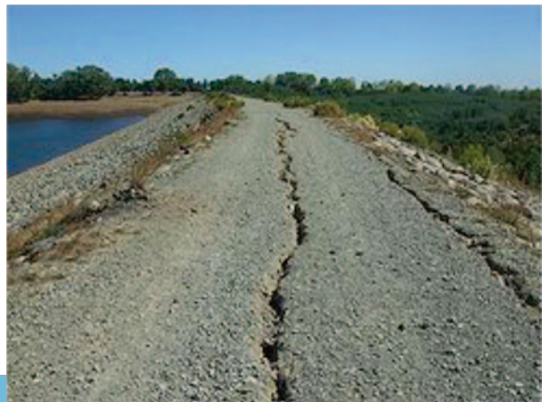
Fig. 14 Coihueco Dam -Longitudinal cracks at the crest
