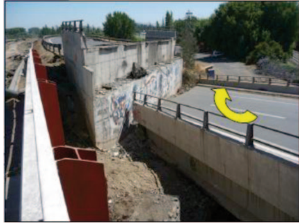
Fig. 26 Collapse of hospital overpass
