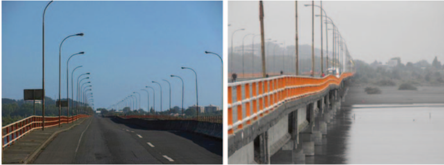
Fig. 21 Settlements along Juan Pablo II Bridge with no evidence of horizontal displacements
