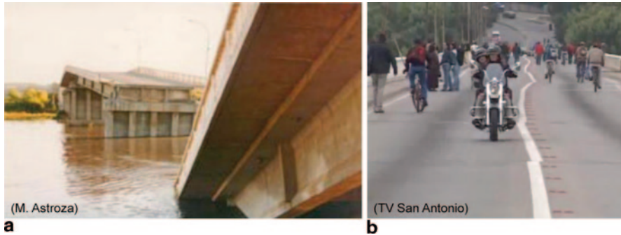
Fig. 25 Liquefaction-induced damages in Lo Gallardo Bridge: a Collapse after the 1985 earthquake. b Misaligned of new bridge after the 2010 Chile earthquake
