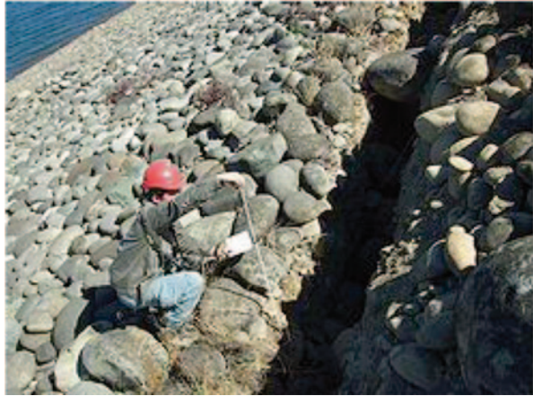
Fig. 15 Coihueco Dam- Downward slope movement at the upstream shoulder
