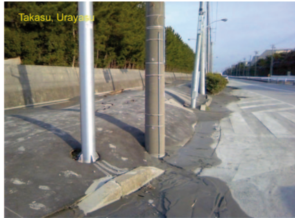
Fig. 20 Heaving of a foot-way in the Takasu district of Urayasu City
