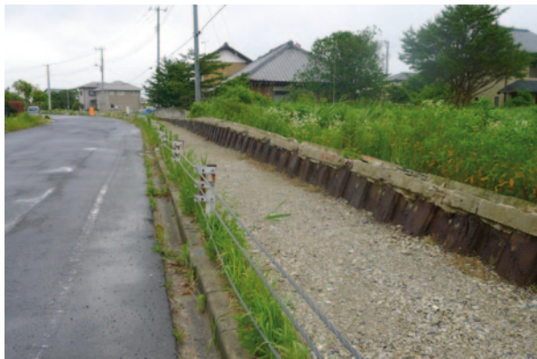
Fig. 17 Lift up and outward distortion of the buried sheet pile row accompanied by lateral displacement at location B in Fig. 13—A view to the eastsouth
