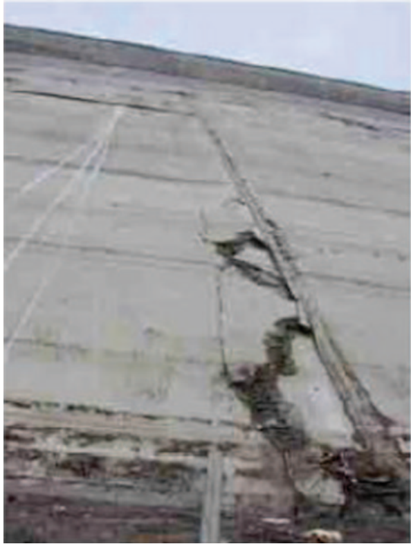
Fig. 25 Zipingpu dam joint damages. (after Chen 2008)
